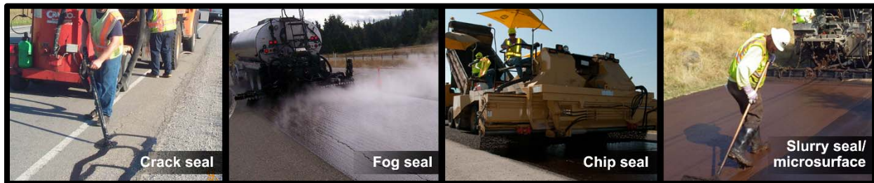
Figure 8: Examples of capital preventive maintenance treatments, (from left) crack seal, fog seal, chip seal, and slurry seal/microsurface.
