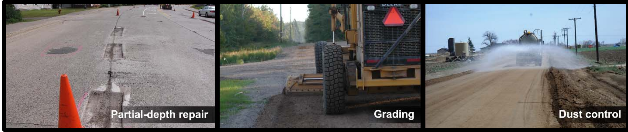
Figure 9: Examples of capital preventive maintenance treatments, cont'd, (from left) concrete road prepared for partial-depth repair, gravel road undergoing maintenance grading, and gravel road receiving dust control application (dust control photo courtesy of Weld County, Colorado, weldgov.com).
