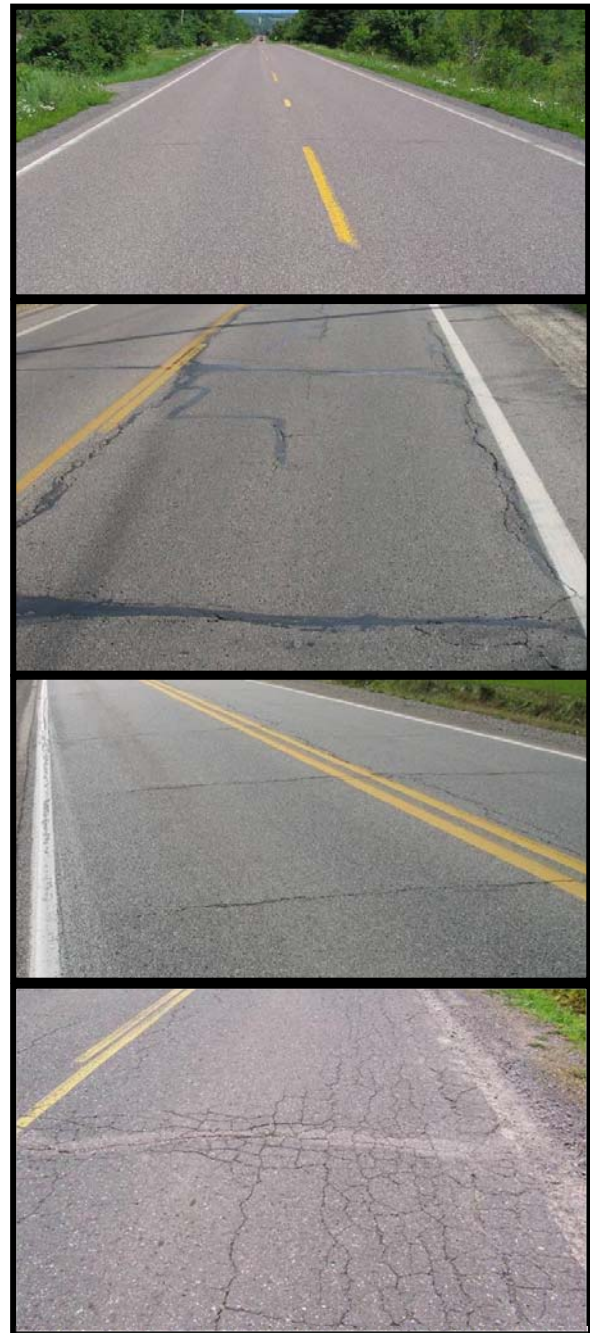
Figure 4: Top image , PASER 8 road that is considered “good” by the TAMC exhibit only minor defects. Second image , PASER 5 road that is considered “fair” by the TAMC. Exhibiting structural soundness but could benefit from CPM. Third image , PASER 6 road that is considered “fair” by the TAMC. Bottom image , PASER 2 road that is considered “poor” by the TAMC exhibiting significant structural distress.
