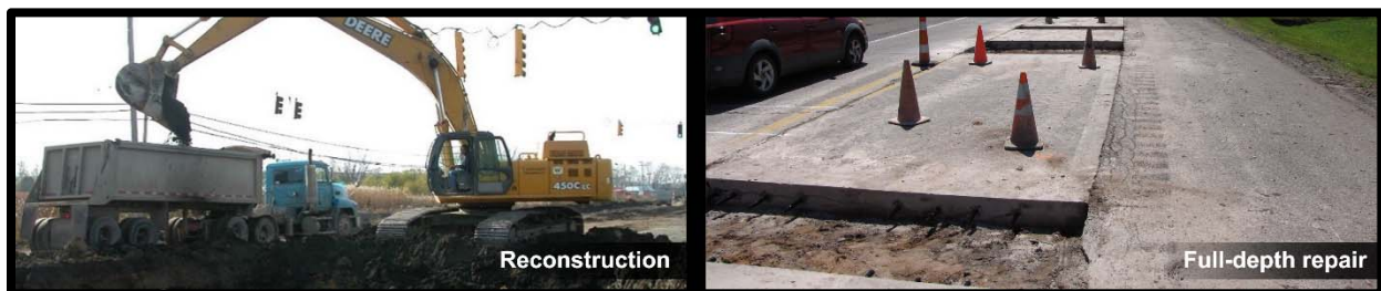
Figure 6: Examples of reconstruction treatments, (left) reconstructing a road and (right) road prepared for full-depth repair.
